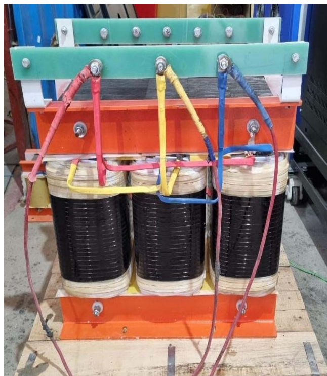
Fig.5 60 kVA ISOLATION TRANSFORMER
