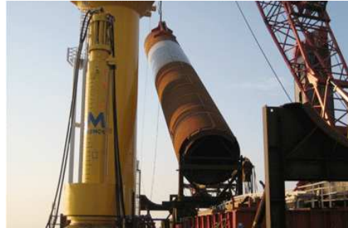
Figure 1–7 Monopile foundation for the Horns Reef II offshore wind farm. (Doe Ringo 2014)
