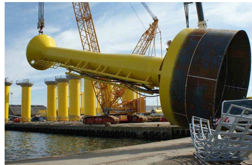
Figure 1–8 Monopod bucket used as foundation for the Mobile Met Mast at Horns Reef II offshore wind farm. (Bakmar 2009)
