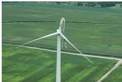
Figure 1 – Wind turbine with a critical blade failure, from [2]
